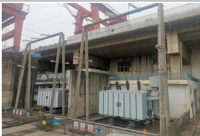
升压站现有主变
